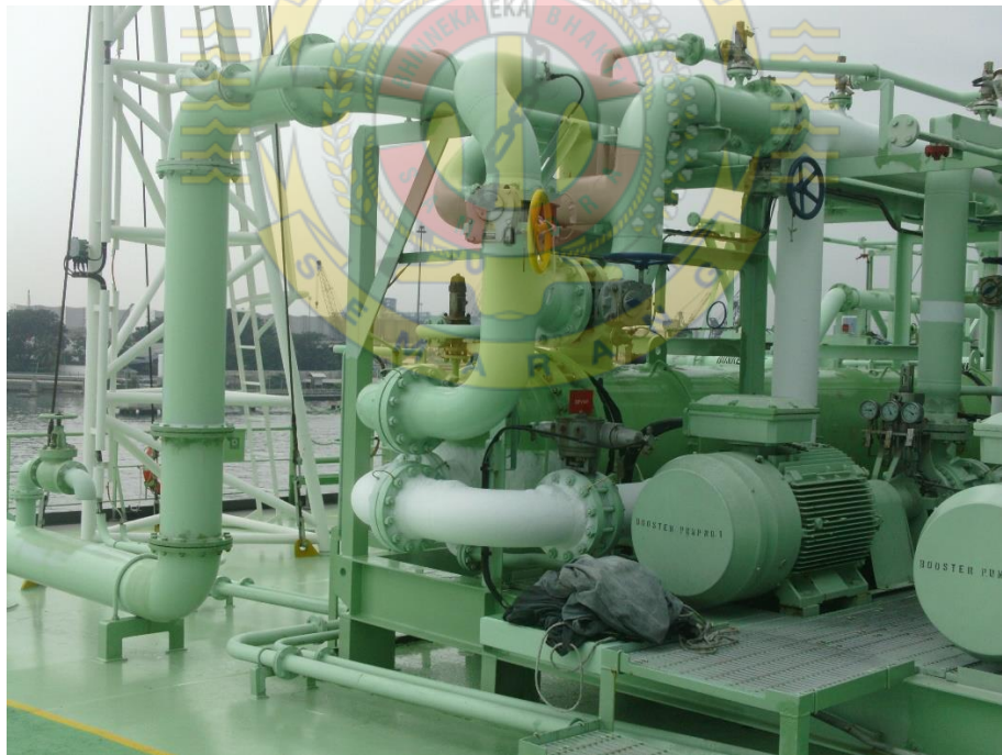
Cargo heater di kapal MT. Gas Widuri
