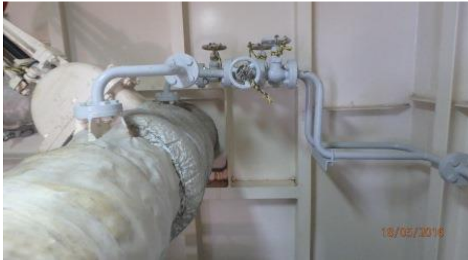
PICTURE CARGO MANIFOLD AIR BLOW LINE VALVE MT. JAYA OCEAN
