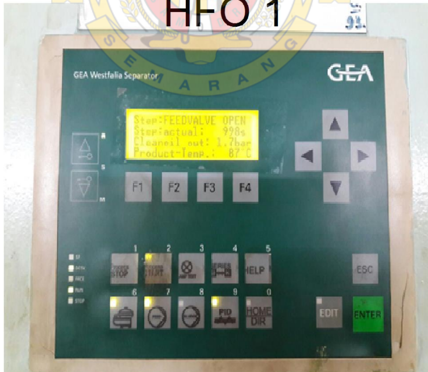
Gambar 4.9 HFO setting temperature panel
