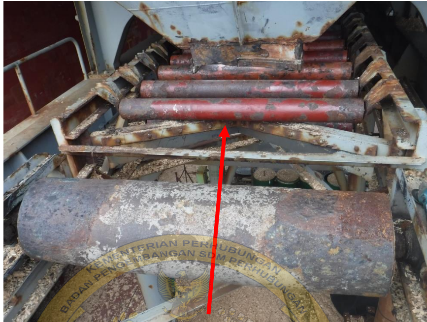
Roller Conveyor Damage
