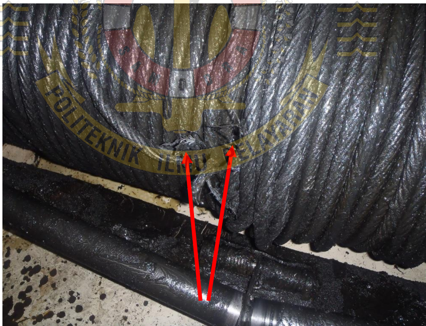
Wire Rope Broken
