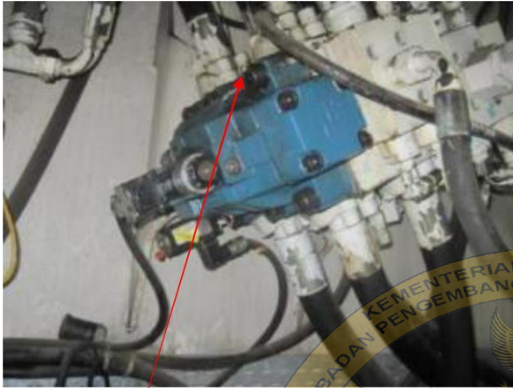
Leaking from vale block.
