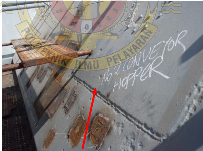
Hopper Conveyor Damage
