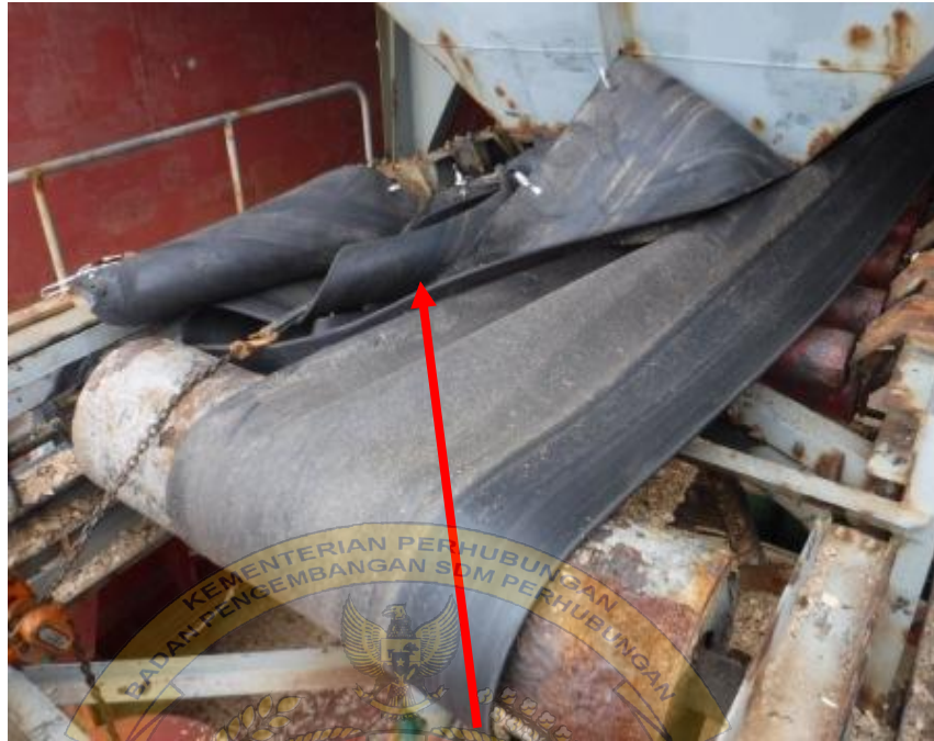
Feeder Conveyor Belt Damage
