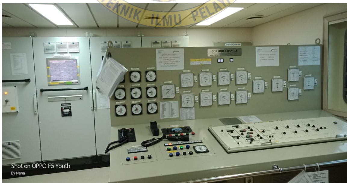
Gambar 4.6 Cargo Control Room (CCR) Kapal VLGC Pertamina Gas 1
