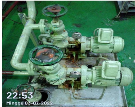
Gambar 2. 10. Deck Water Seal Pump
