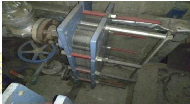
Gambar 2. 4 Lo Cooler type plate KM.Binaiya
