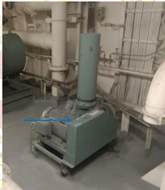
Gambar 2. 7 Root Blower for Unloading Sumber: Dokumen Penelitian (2024)
