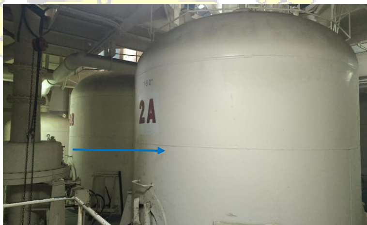
Gambar 2. 4 Cellar Tank Sumber: Dokumen Penelitian (2024)
