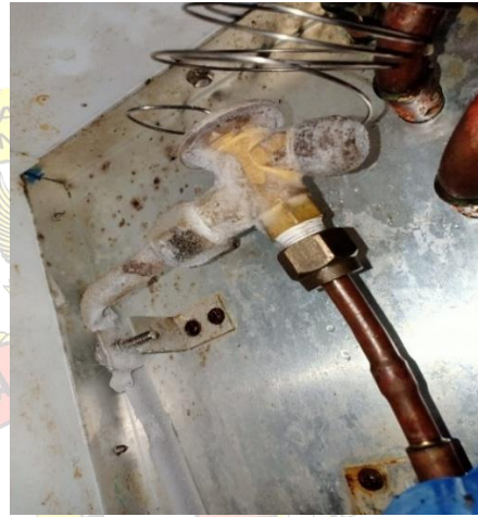
Gambar 2.4 Thermostatic expansion valves
