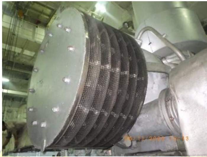
Gambar 2. 4 Air filter silencer (Sumber : Dokumen pribadi)
