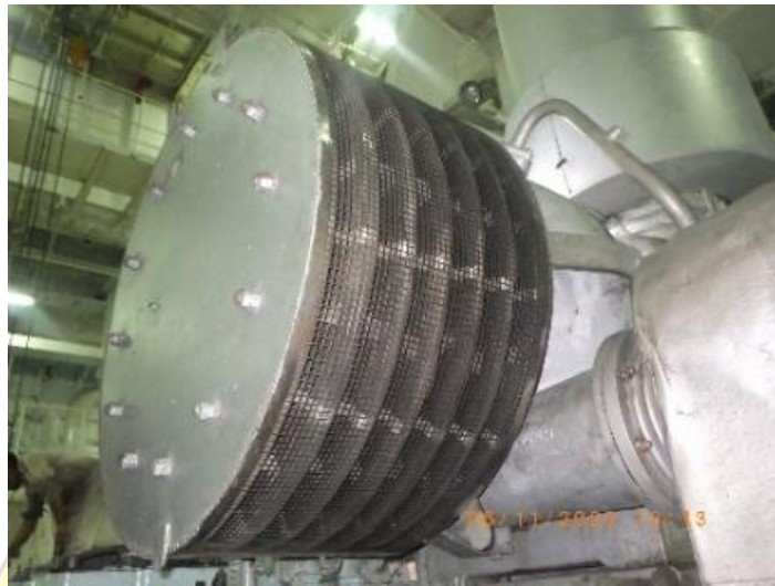
Gambar 2. 4 Air filter silencer (Sumber : Dokumen pribadi)
