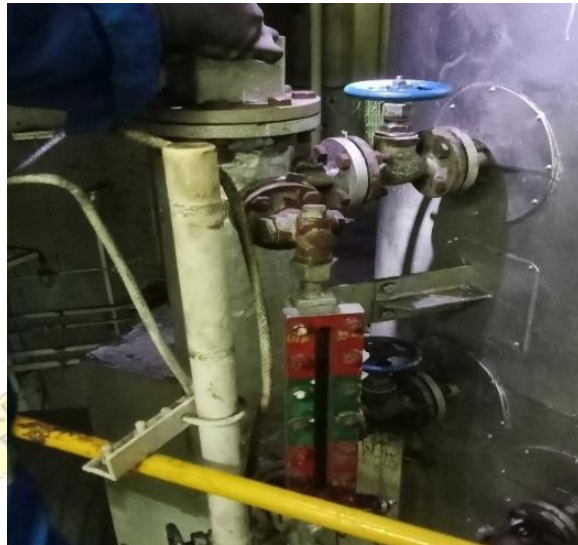
Gambar 2. 7 Water Level Gauge
