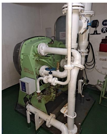
Gambar 2. 1 Fresh Water Generator
