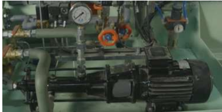
Gambar 2. 13 Sludge Dossage Pump
