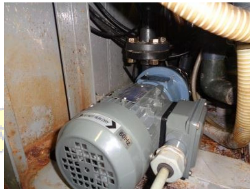
Gambar 2. 10 chemical transfer pump Sumber : manual book kuraray
