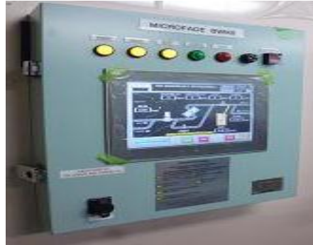
Gambar 2. 7 main control unit BWMS
