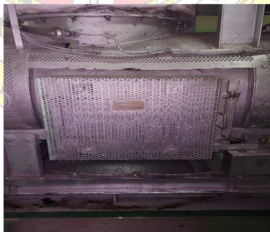
Gambar 2.6 Ash Removal Door and Charging Door Sumber: Data Pribadi
