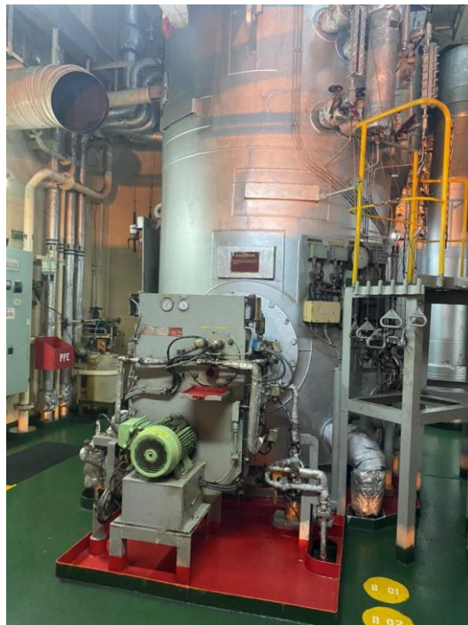
Gambar 2.3 Auxiliary Boiler Sumber : (Dokumentasi penelitian)
