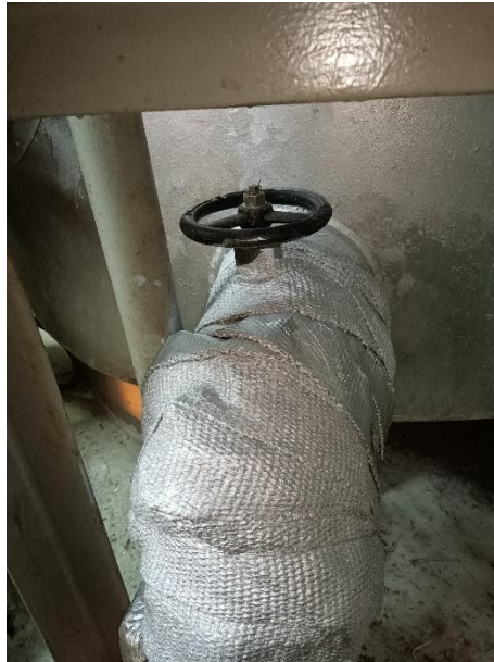
Gambar 2.6 Main steam valve Sumber : (Dokumentasi penelitian)
