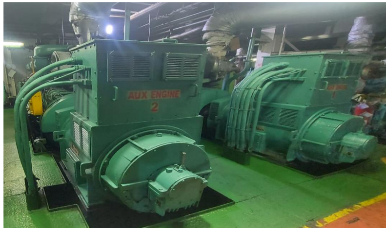
Gambar 2.4 Mesin Diesel Generator Sumber : Data penelitian, 2023
