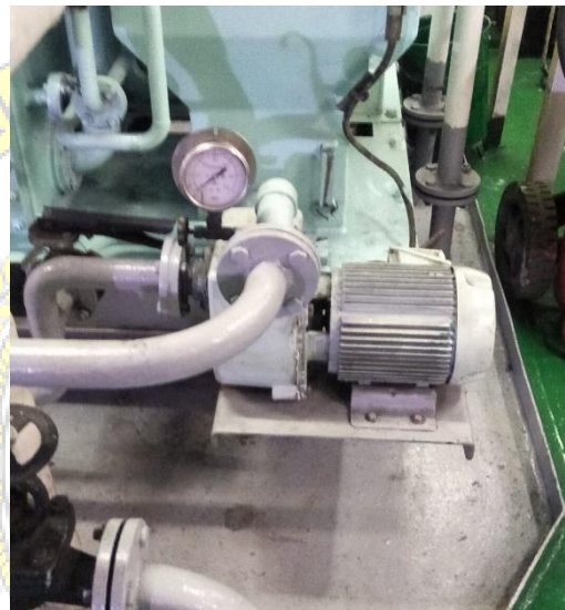
Gambar 2.8. Discharge Pump Sumber : Data Penelitian, 2022
