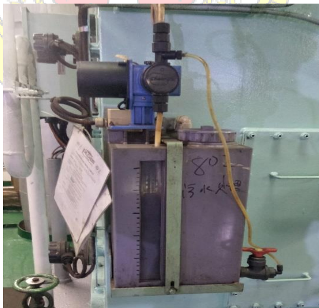
Gambar 2.6. Chemical pump dan Chemical tank
