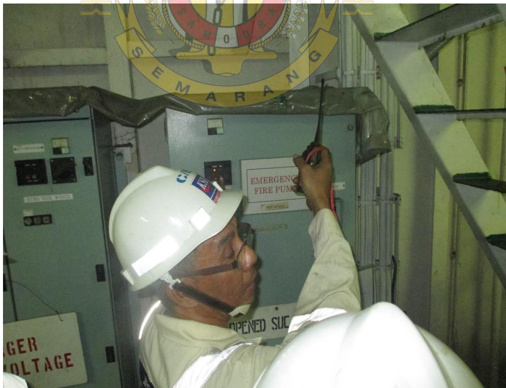
Gambar 14 Emergency Fire Pump Test
