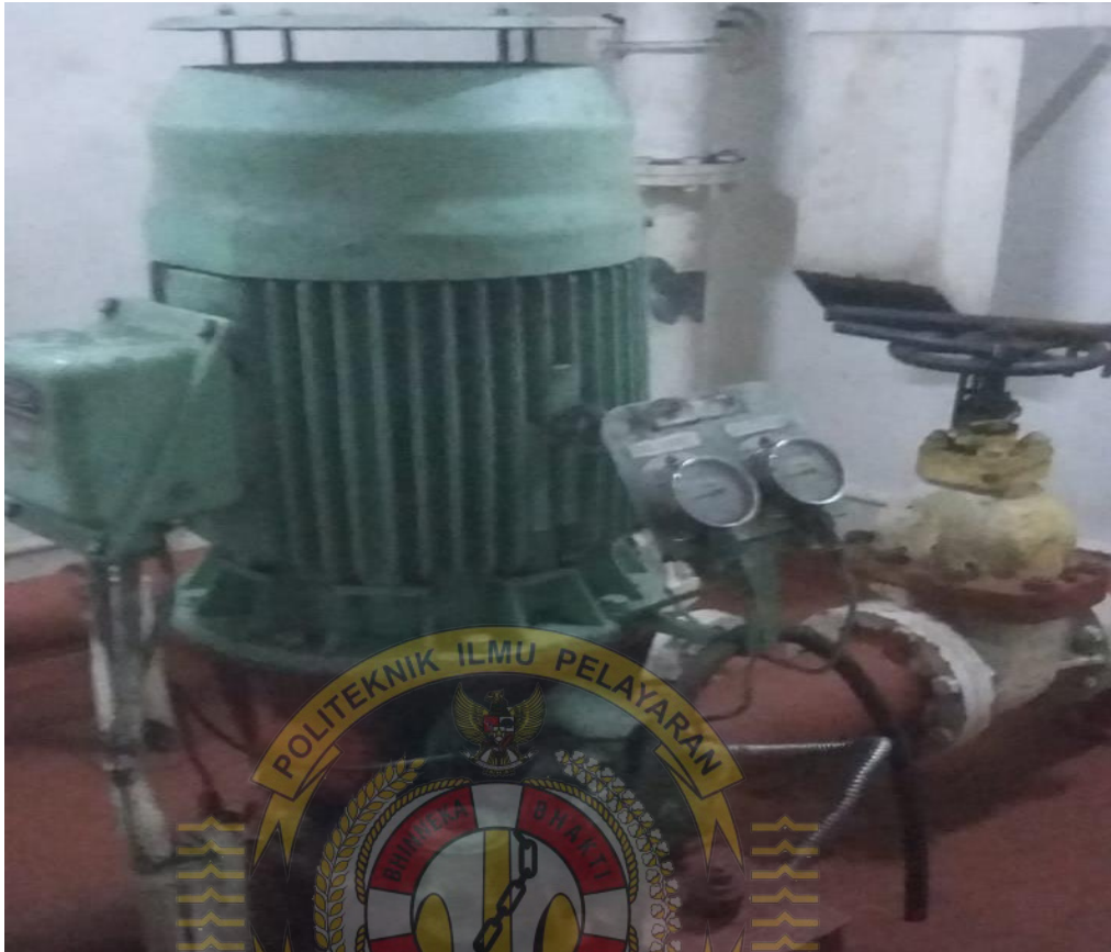
Gambar 14 Emergency Fire Pump
