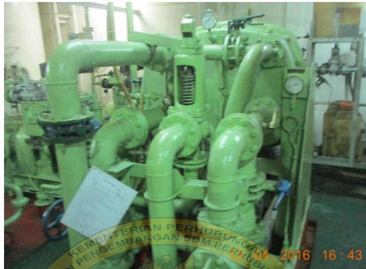
Fresh Water Generator Safety Valve
