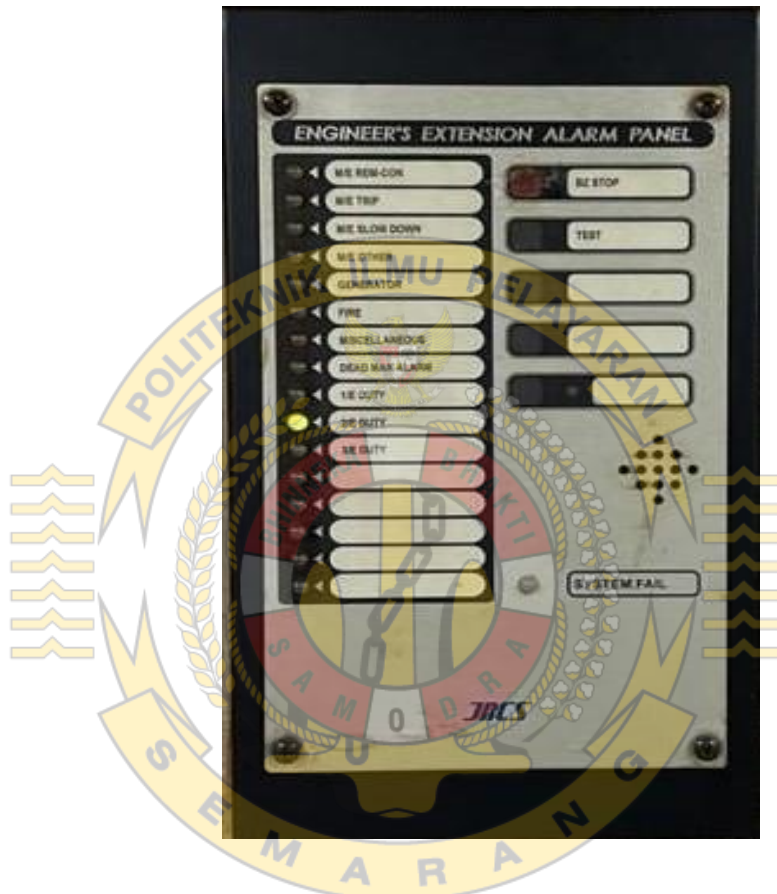
Gambar 2. 2 UMS Alarm Panel
