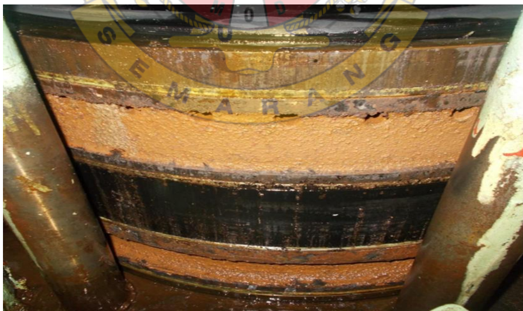
Kondisi bocor jacket cooling sistem main engine
