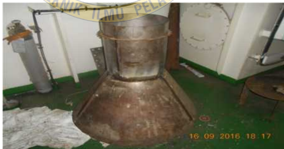
Gambar 2.2. Ruang Bakar Inert Gas Generator
