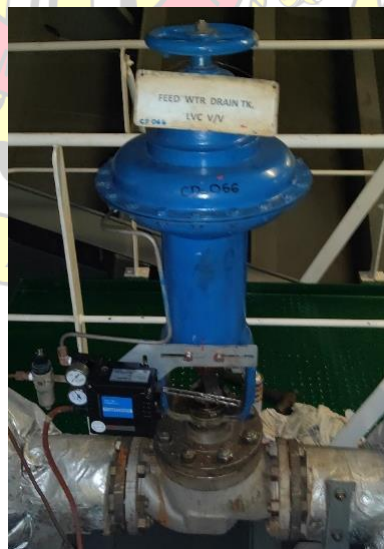
Gambar 2.11 Feedwater Drain Tank Level Control Valve
