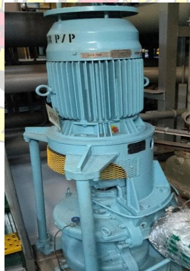
Gambar 2.10 Navigation Drain Pump
