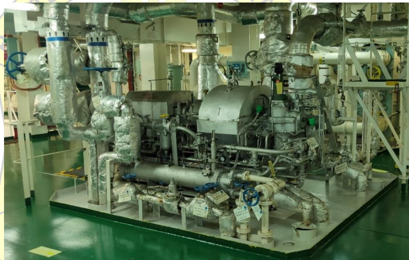
Gambar 2.7 Main Feed Water Pump Turbine
