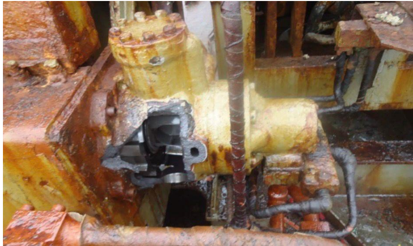
Lampiran 5 kondisi Hydraulic oil pump pecah
