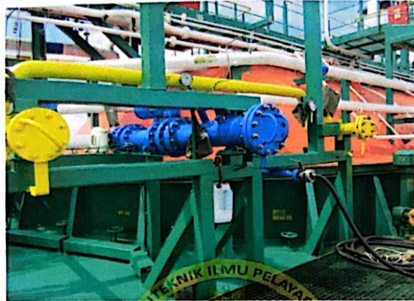
Gambar: Manifold LPG/C Gas Arjuna.
