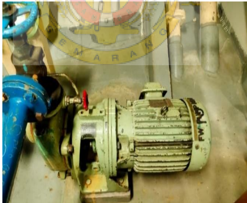
fresh water pump
