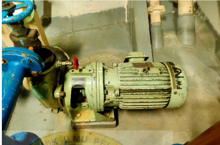
Gambar 2. 5 Fresh water pump
