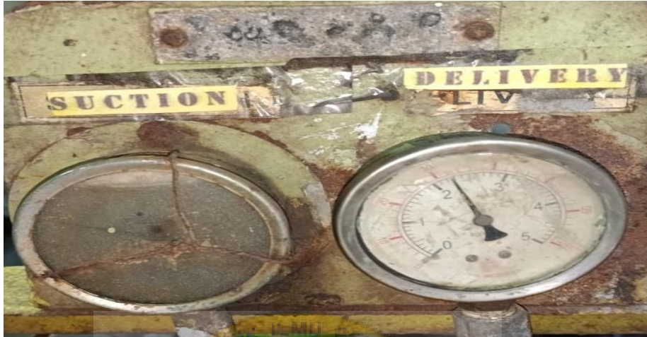
Tekanan main cooling sea water pump
