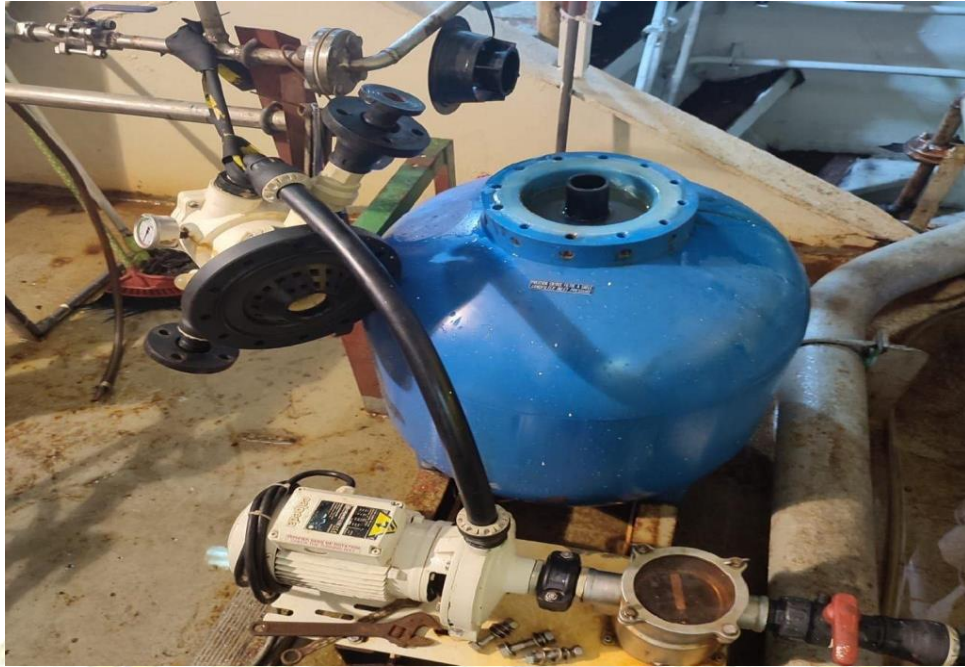
Gambar 8 : Maintenance Sand Filter
