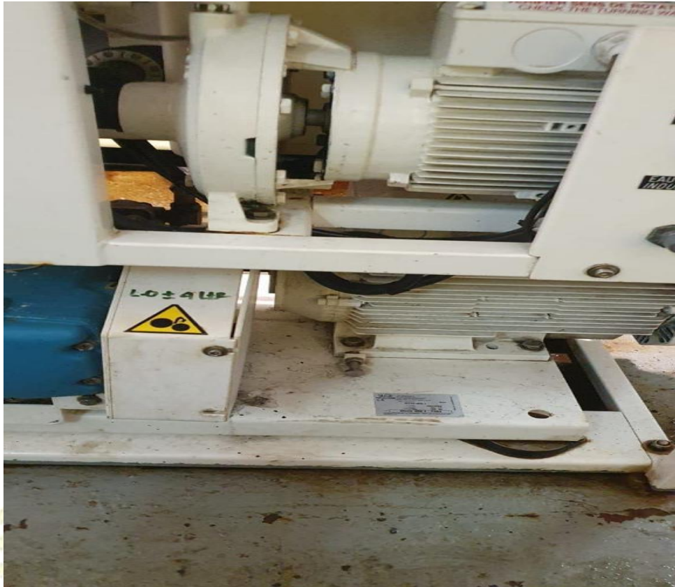
Gambar 20 : Pompa High Pressure
