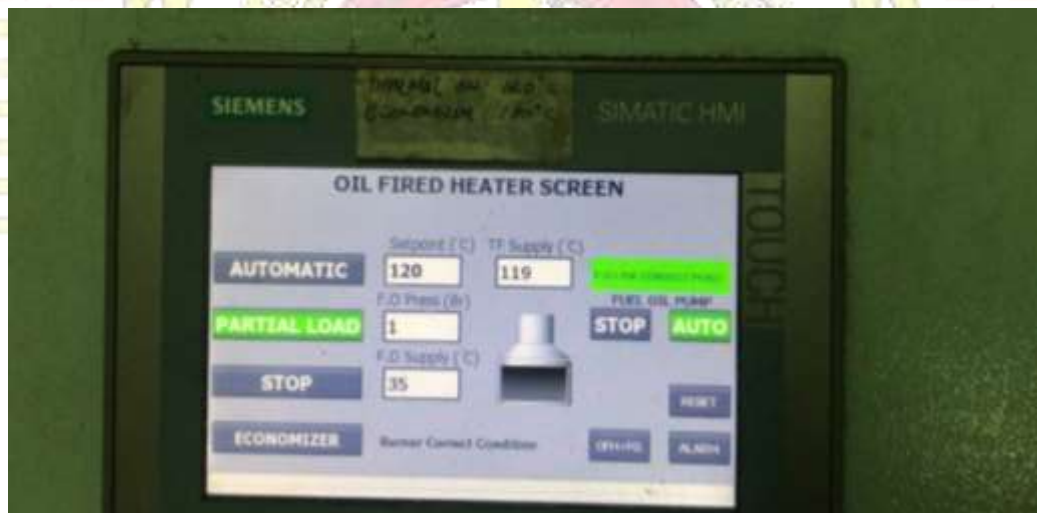
Gambar 10 Panel Thermal Oil Heater 2
