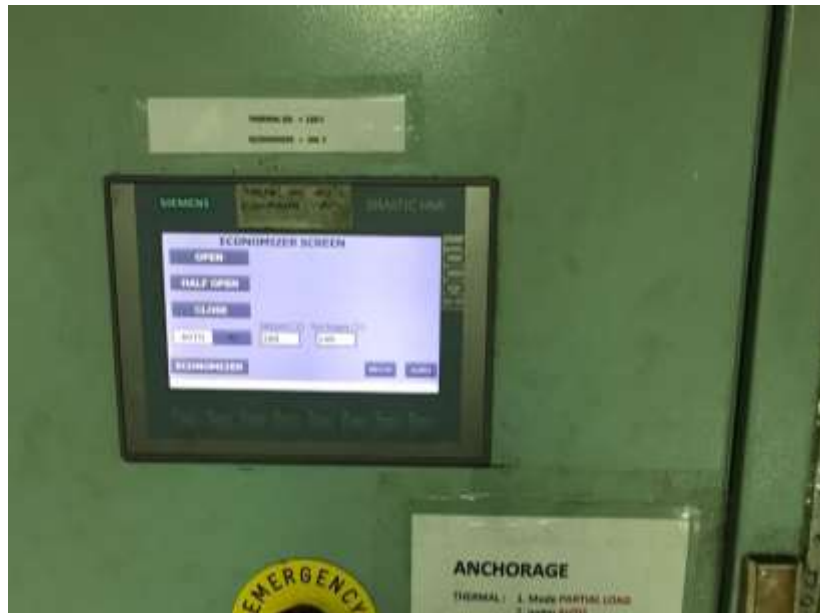
Gambar 9 Panel Thermal Oil Heater 1
