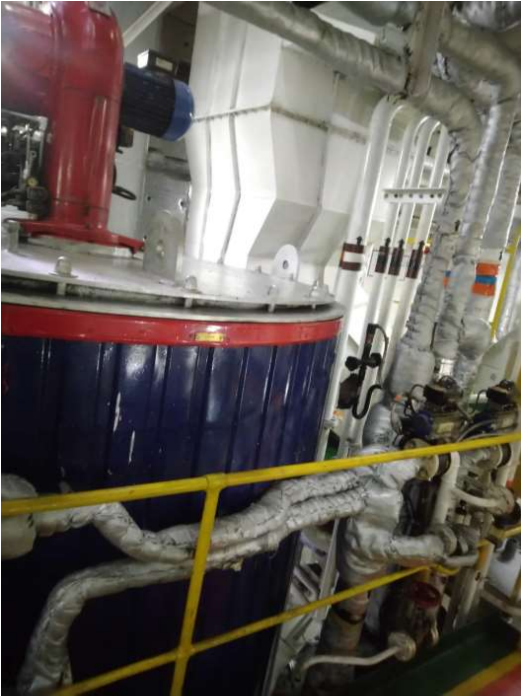
Gambar 8 Thermal Oil Heater
