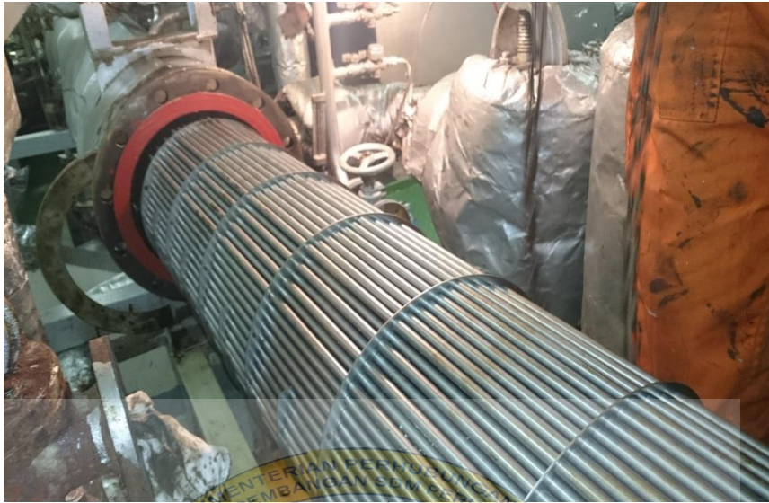
Gambar 2.6 main fuel oil heater
