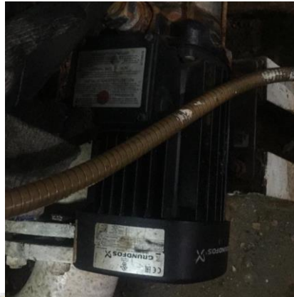
Gambar 2.4 Fresh Water Pump
