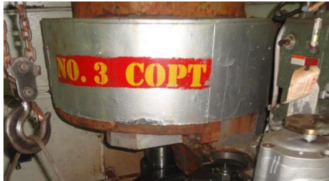
Gambar 2.3 Casing Cargo Oil Pump Turbine no.3
