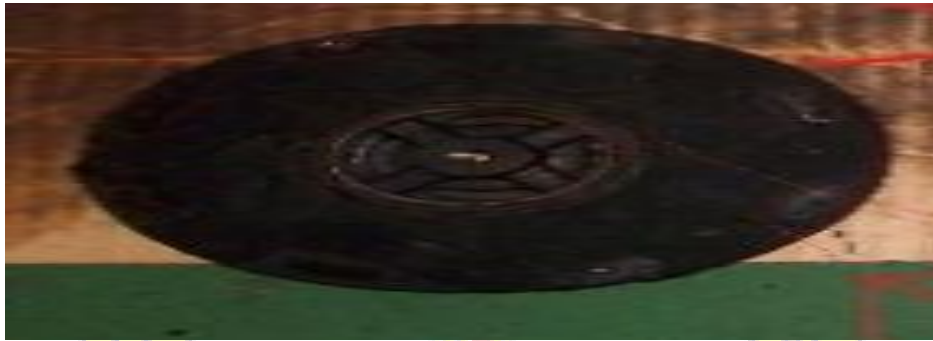
Kondisi Low Pressure Valve Main Air compressor
