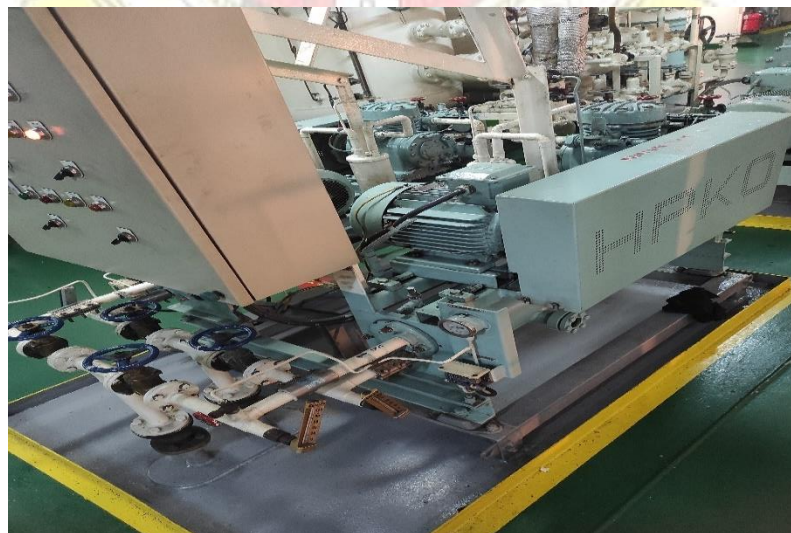
Gambar 2.17 provision refrigeration plant
