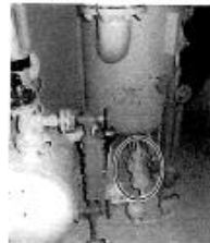
Open drain valve for mist separator
