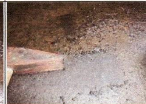
Layer of rust could be removed by fine chipping, black color is bare metal.
