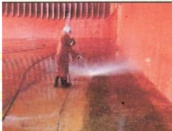
Layer of rust removed by high pressured F.W Jet on tank top.
