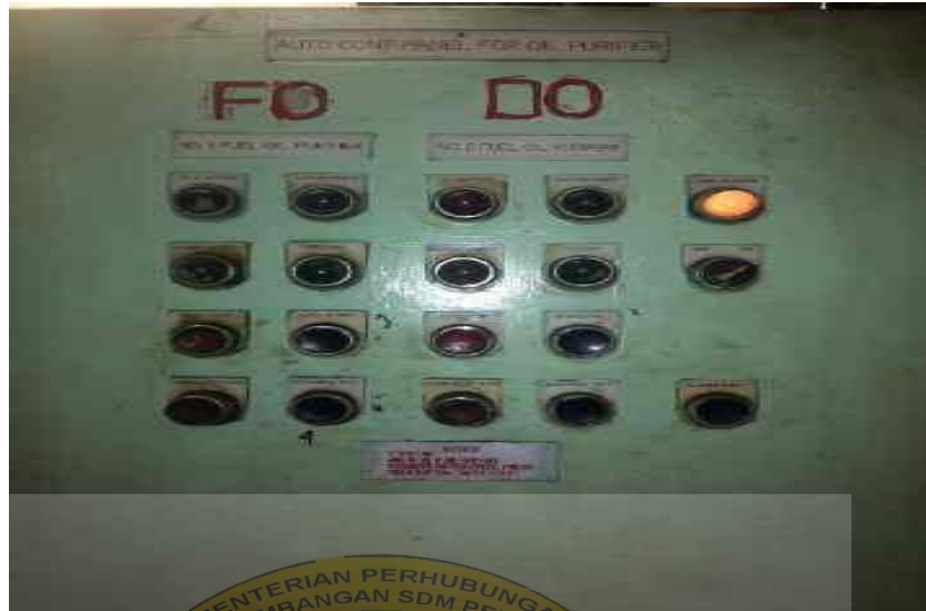
Gambar : Panel MDO Purifier
