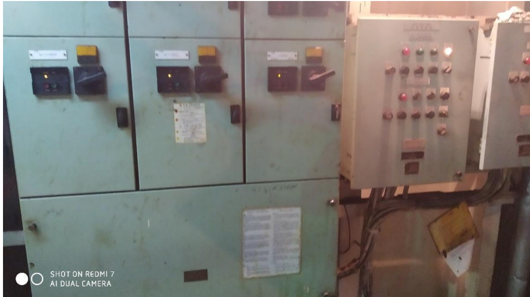
Panel pada feed water pump auxiliary boiler steam
