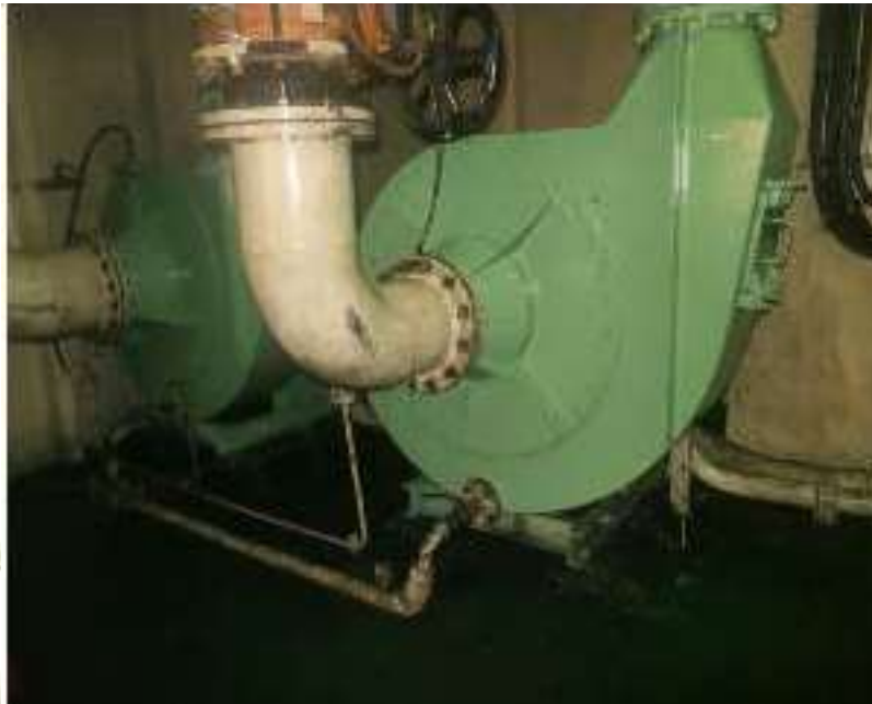
Gambar 2. 2 Blower Inert Gas System
