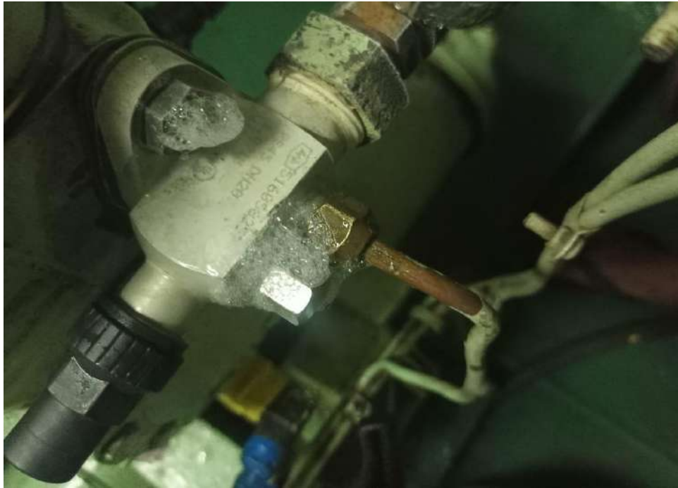
Kebocoran pipa hisap compressor MT. RATU RUWAIDAH
