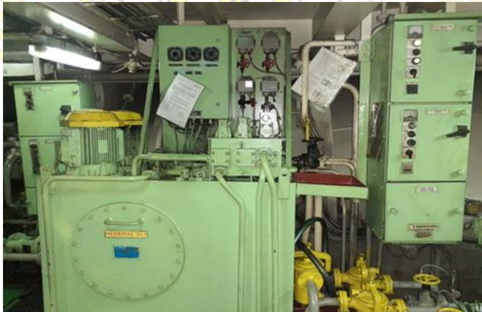
Gambar 4.2 Power pack hydraulic CPP
