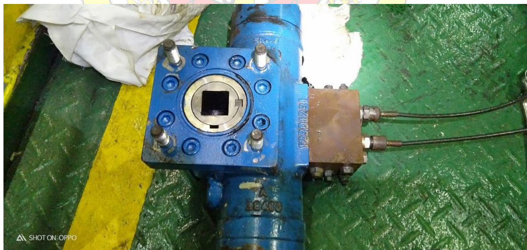
PENGECEKAN ACTUATOR VALVE
