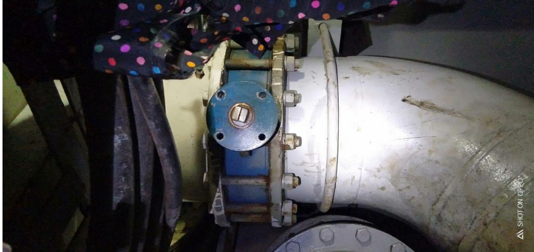
BUTTERFLY VALVE YANG STUCK CLOSED
