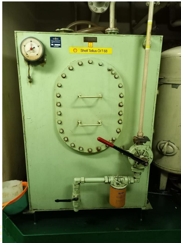
Storage tank steering gear
