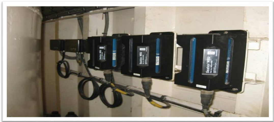
Figure 22. MRU's Located Forward in the Cement Compartment
