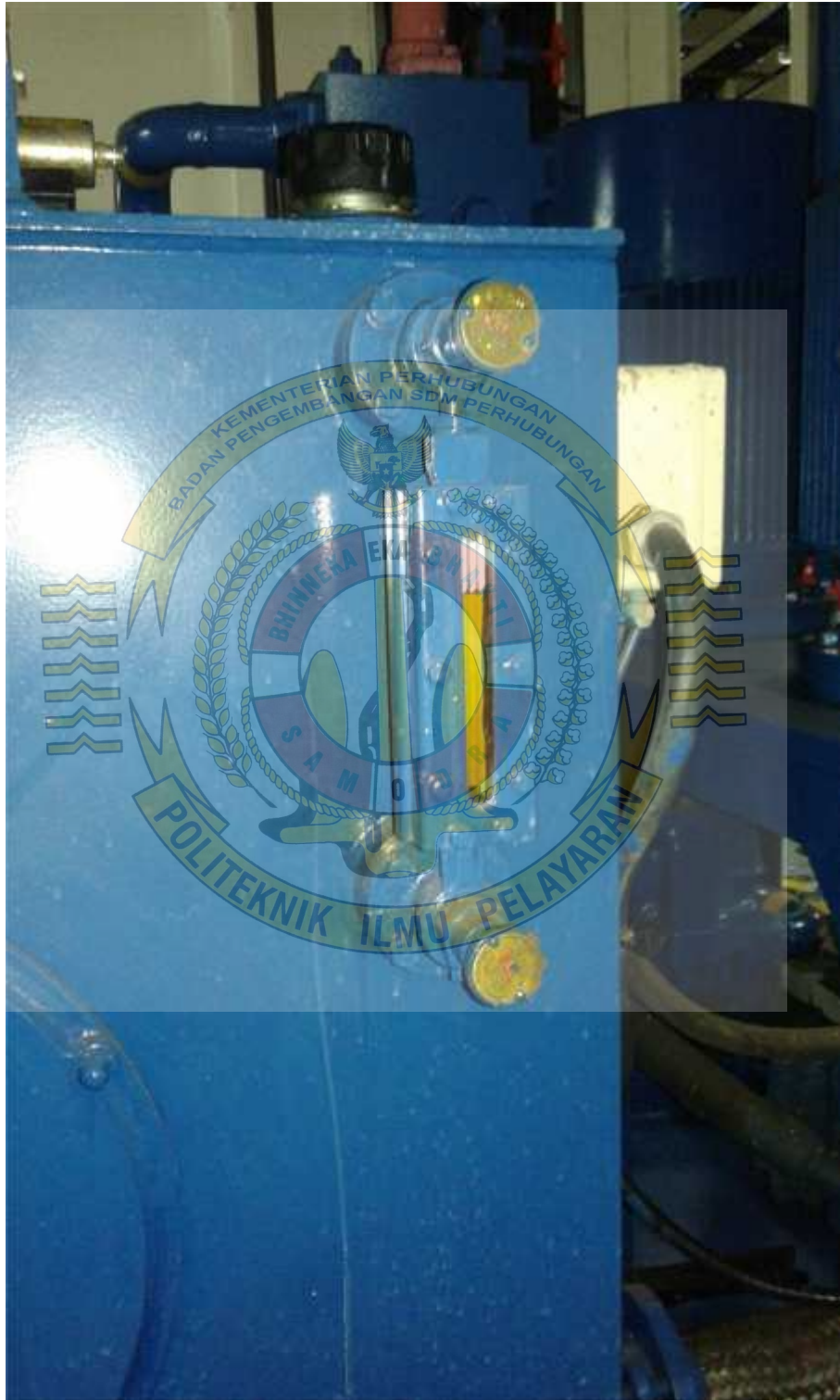
Lampiran 6 : Anchor Handling and Towing Winch Hydraulic Oil Tank
