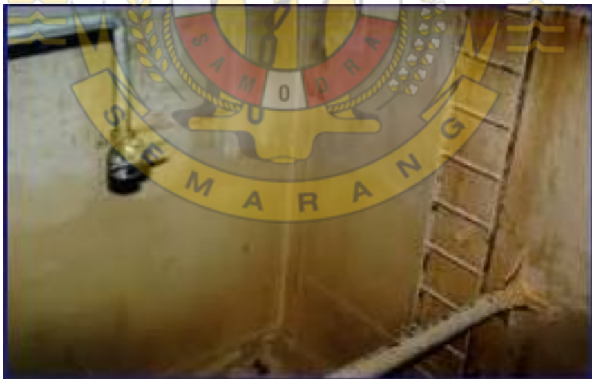
Gambar Lampiran 4 Kondisi Tanki ballast no 6 sesudah cleaning
