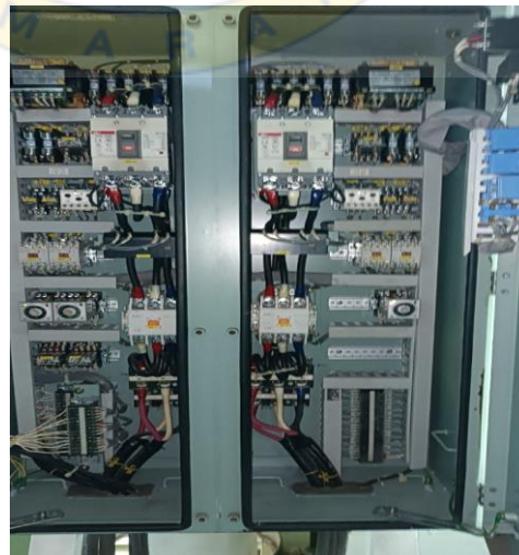
3. Gambar panel auxiliary blower mesin induk
