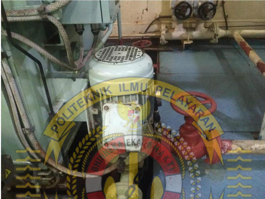
Gambar kondisi pompa pembuangan sewage treatment plant
